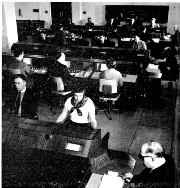
A general view of the new cordless switchboards in Fleet Building. Calls are connected in the order in which they are received.
