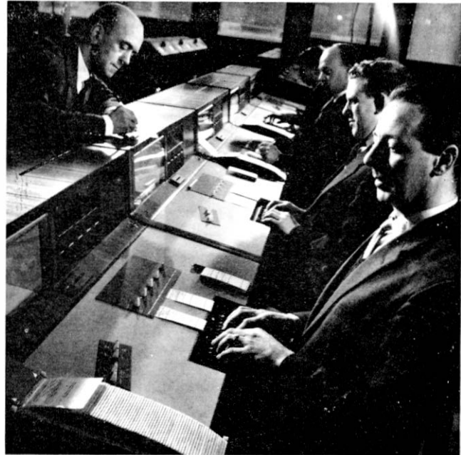
A view of the positions dealing with calls routed via cable circuits. Seen in the background are the radio telex positions.
