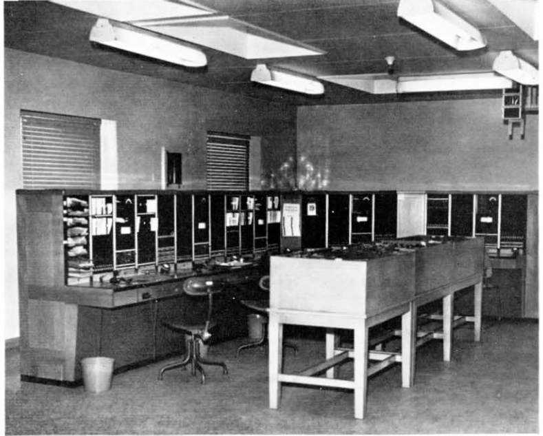
A general view of the test room at the new Altrincham Exchange. Note the roof light apertures in the ceiling.
