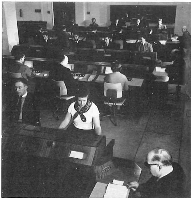
A general view of the new cordless switchboards in Fleet Building. Calls are connected in the order in which they are received.
