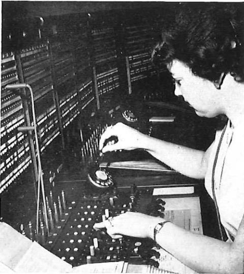
An operator at the Monarch Telephone Exchange, London, goes through the procedure of dialling a distant number.
