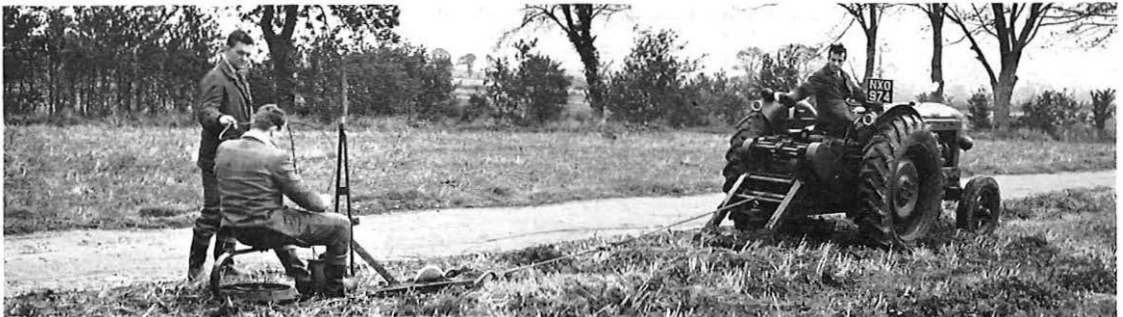
Standard Post Office moleplough in use with tractor mounted winch and sprag
