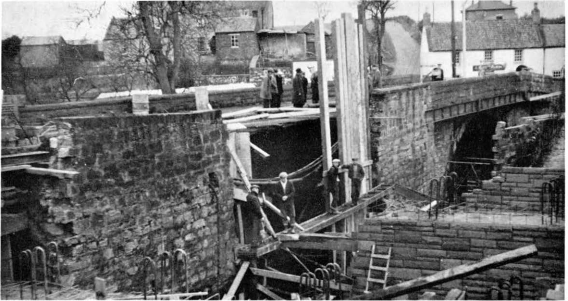
Fig. 3: Cables damaged during bridge building
