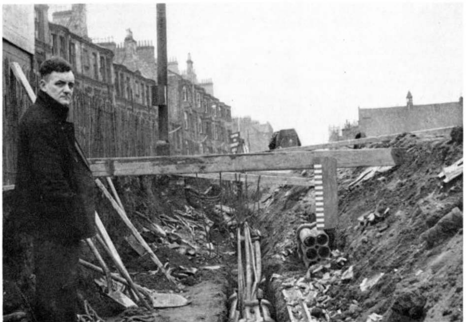
Fig. 4: Shattered 6-way duct
