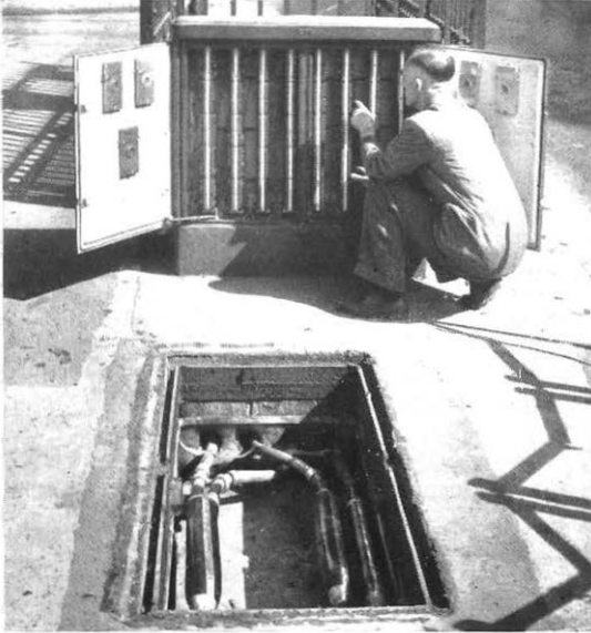
Fig. 2: Interior of cabinet and associated footway jointing box
