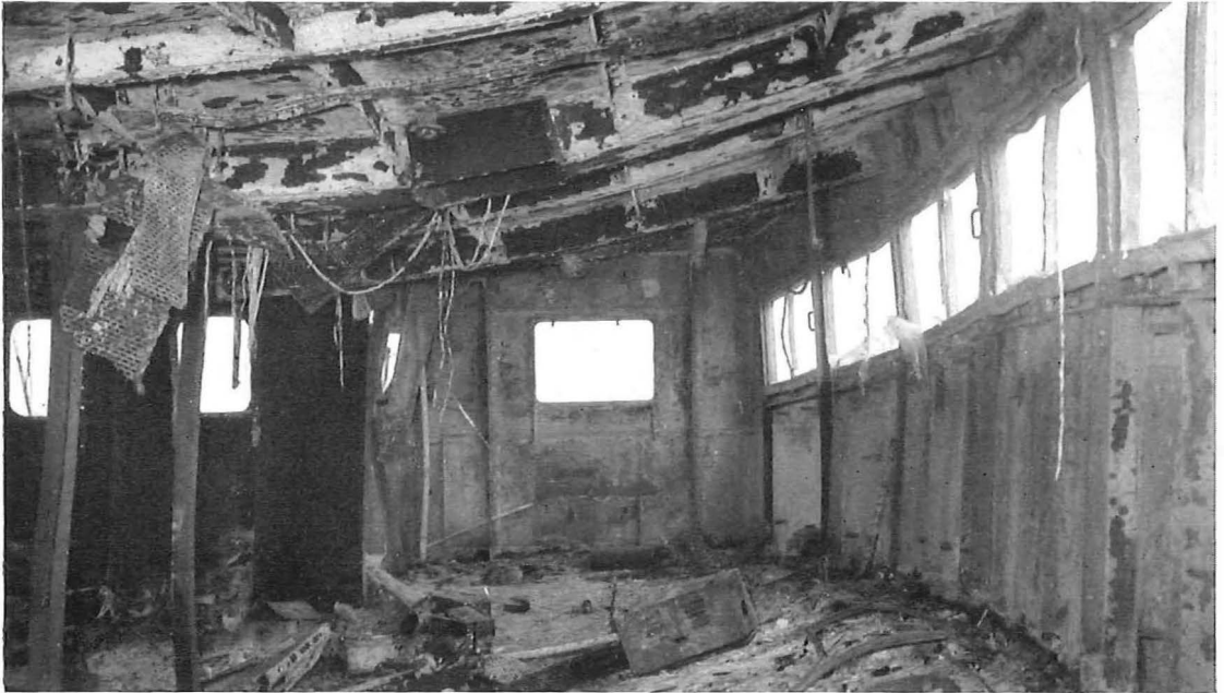
Fig. 3 : Bridge of the Ocean Layer after the fire looking towards the Port side
