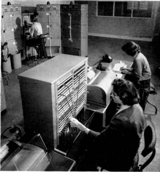
Fig. 4: Supervisory position and jackfield
