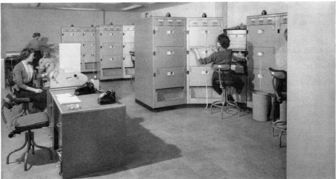
Fig. 3: General view of the tape relay centre
