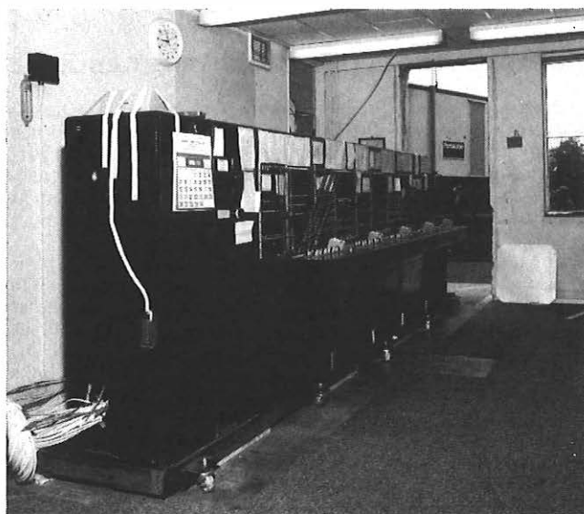
FIG. 2—The PMBX1A switchboard suite with its supporting frame
