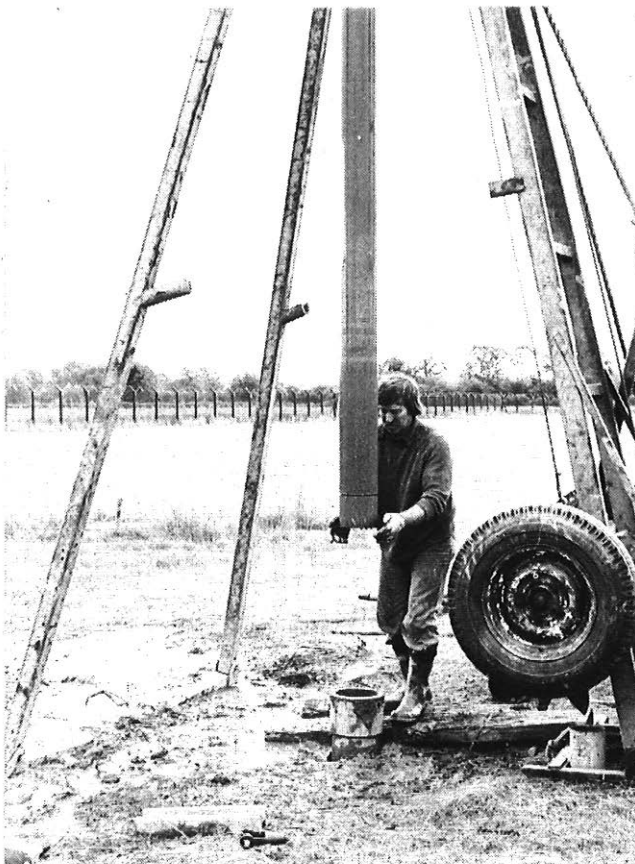
FIG. 4—Site investigation rig showing cutting tool and top of borehole lining tube
