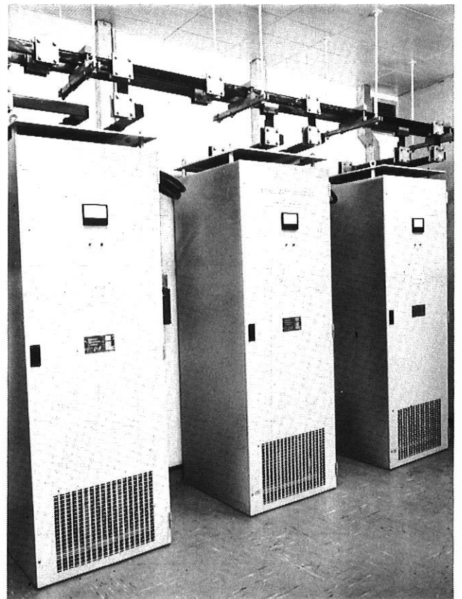
FIG. 4—Suite of three Rectifiers 153B/300 in parallel
