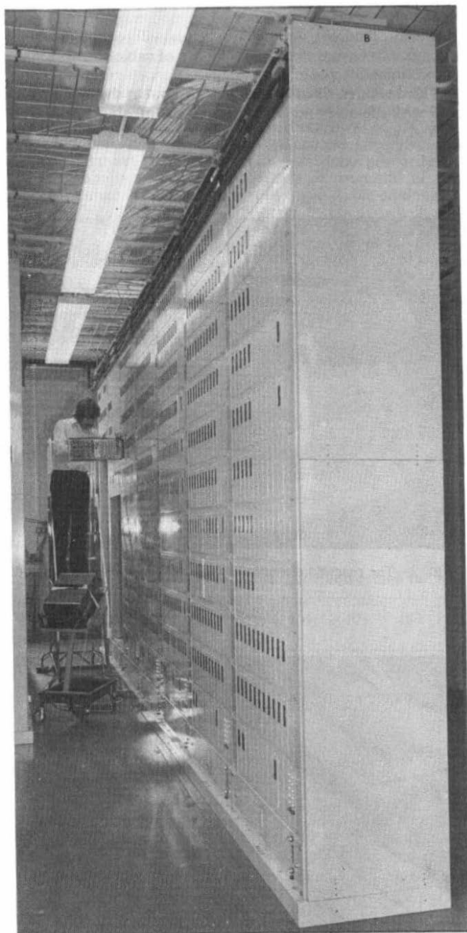
FIG. 6—The Werrington Pentex ERM installation
