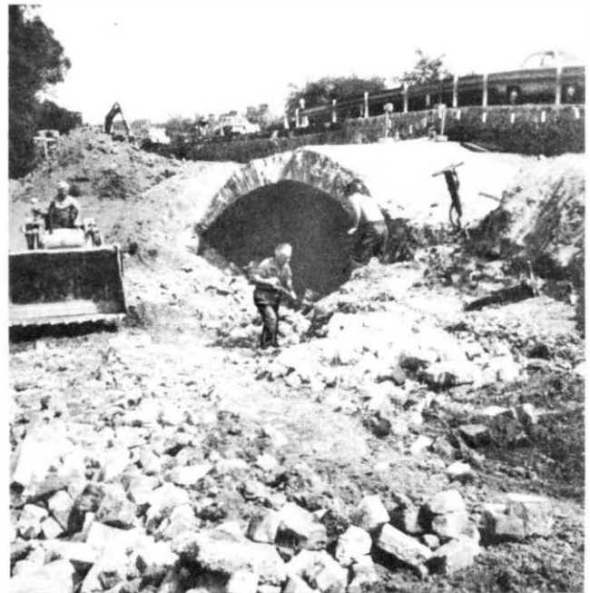
FIG. 3—Demolition of the bridge, with masonry being deposited on the new duct line
