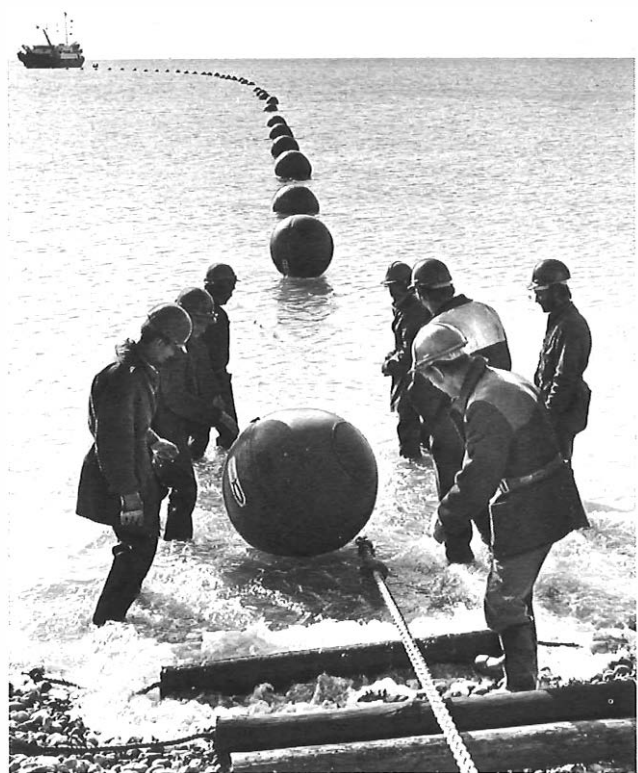
FIG. 4—Preparing to cut away the first float as the cable is brought ashore
