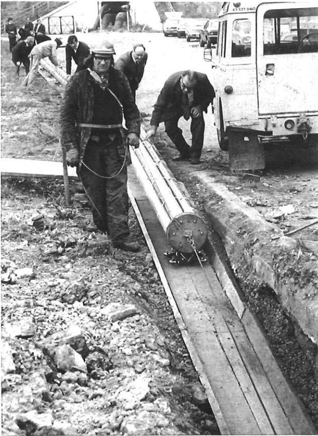
The assembled duct nest being drawn down the ramp to the gas pipe
