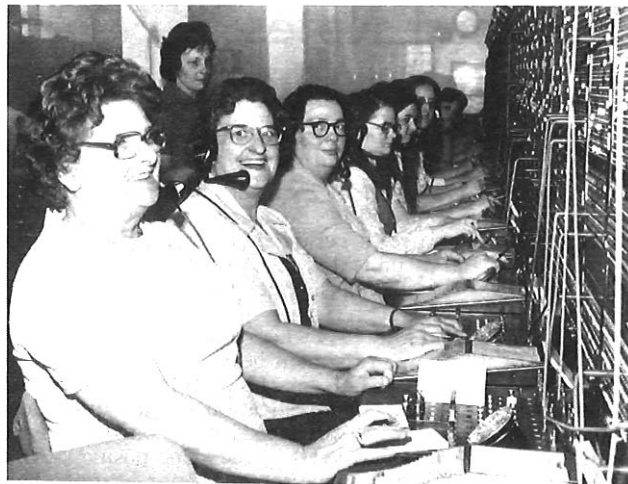
Part of Abingdon's manual board, before conversion
