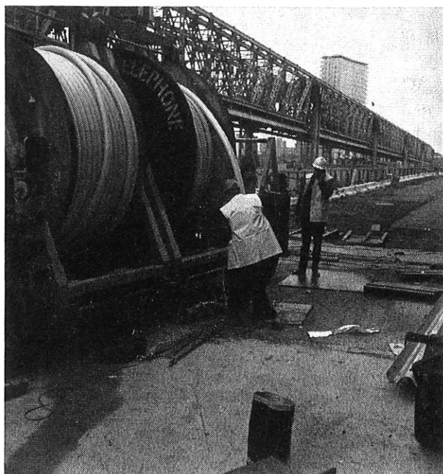
FIG. 2—Cable being fed into ducts, in the main diaphragm below, at the north side of London Bridge
