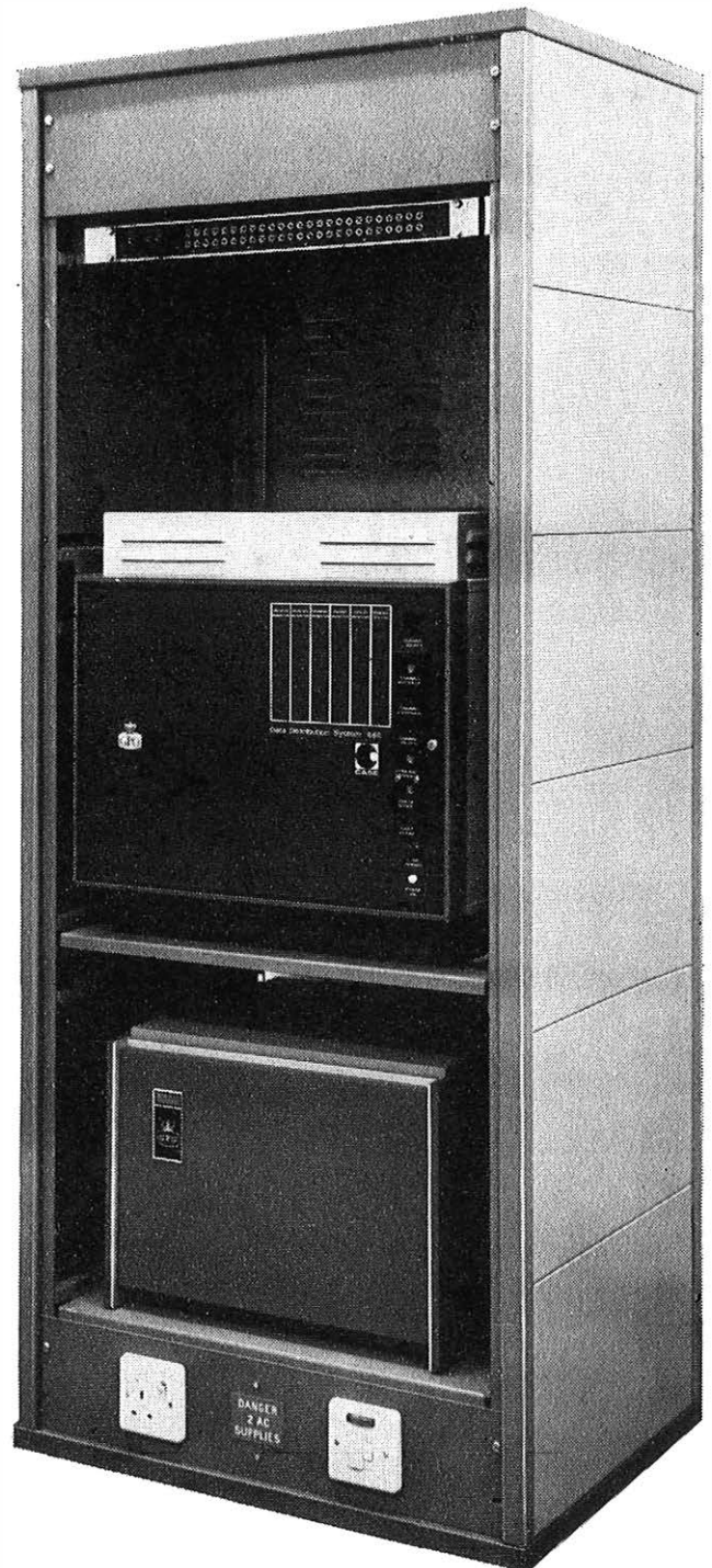
FIG. 2—Installation at the customer's end
