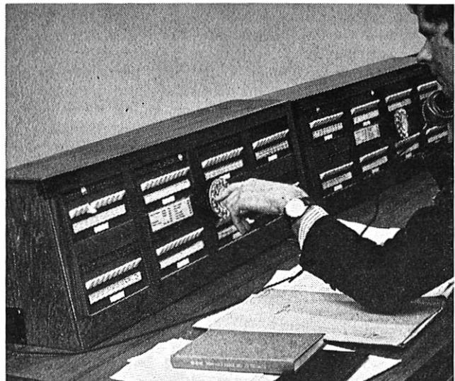
FIG. 1—Ten-line key-and-lamp units installed in a console
