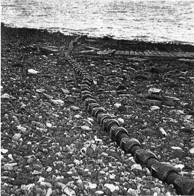
FIG. 1—Cast-iron split-ducts fitted to cable
