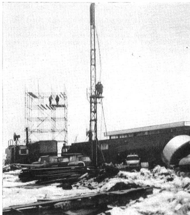
Erection of the scaffold platform with temporary BBC aerial in the foreground
