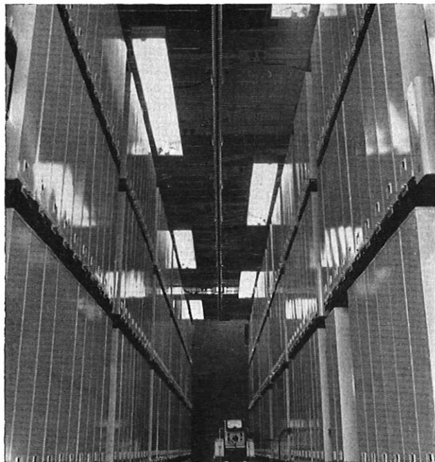
FIG. 7—APPARATUS GANGWAY WITH GRID CABLE-PLATFORM AND WITH NEW LIGHTING FITTING
