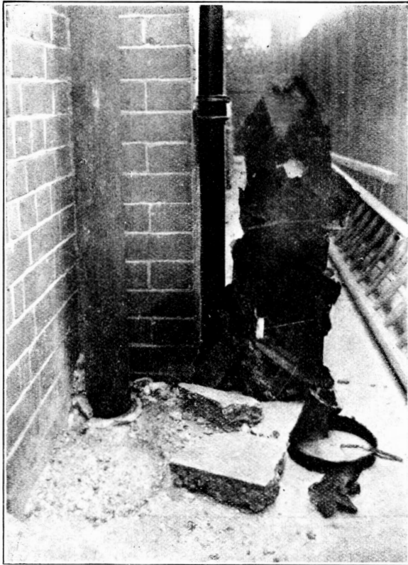
2.--DAMAGED CONCRETE AT BASE OF VENTILATING SHAFT.
