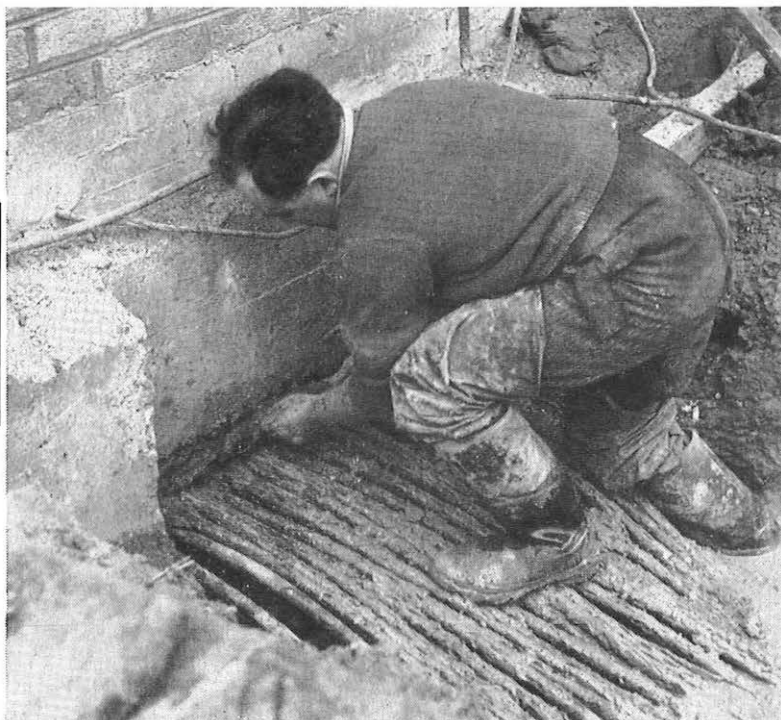
24½" diameter cables passing through duct measuring 36" × 18" × 9" which is completely filled with DENSO MASTIC.
