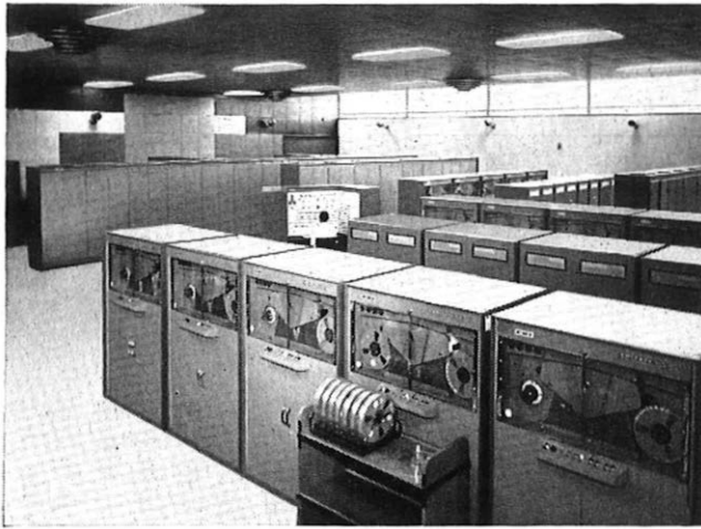
Magnetic tape units in foreground. Conditioned air is supplied by ceiling diffusers
