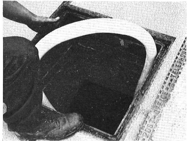
CENTRE OF THE BIGHT OF 1,800 PR., 4 LB/MILE POLYTHENE UNIT-TWIN CABLE ENTERING THE MANHOLE
