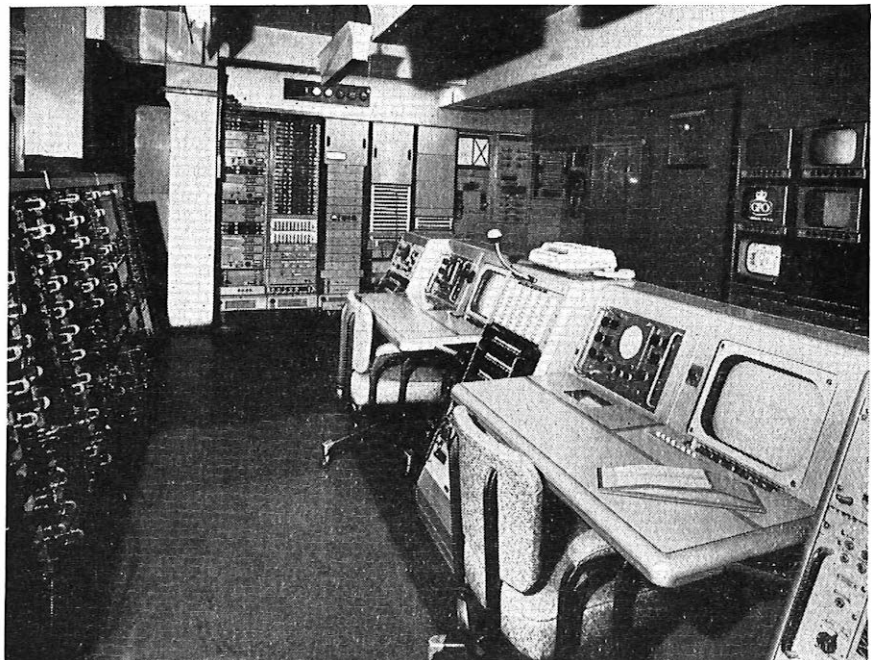
FIG. 1—CONTROL ROOM OF LONDON TELEVISION NETWORK SWITCHING CENTRE
