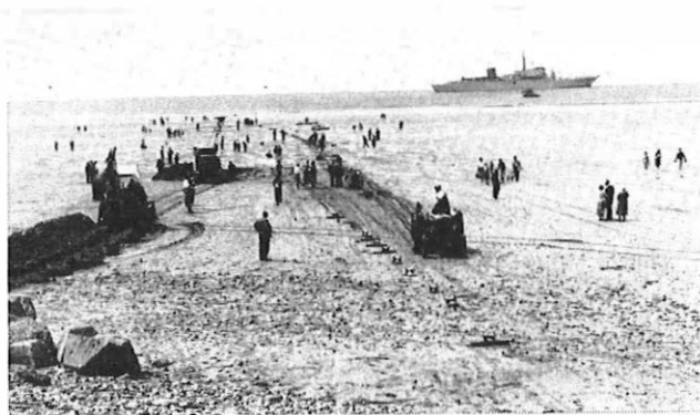
By courtesy of Dempster's Studios, Bielefeld. HAULING ASHORE THE TAT-3 SUBMARINE CABLE AT WIDEMOUTH BAY, CORNWALL.
