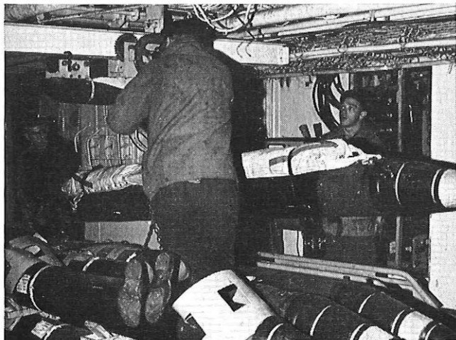
FIG. 3—LOADING THE NEXT REPEATER TO BE LAID ON TO A TROLLEY IN THE CENTRE CASTLE OF MONARCH
