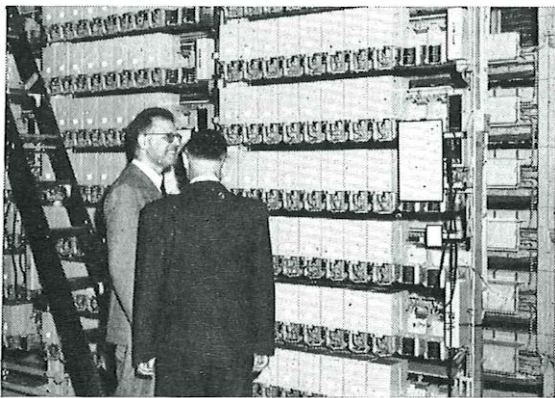
STC equipment in Valletta Central Automatic Exchange
