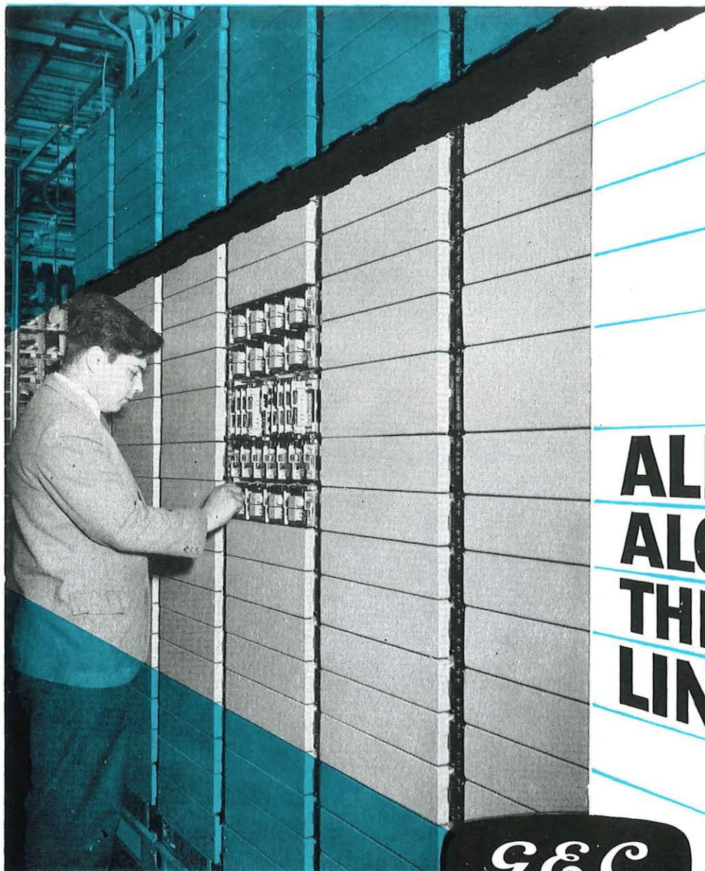
Type 56 transistored channel equipment at Faraday Building.
