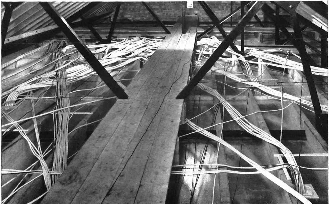
FIG. 1—CABLING ABOVE THE CEILING AT BISHOPS CLEEVE EXCHANGE
