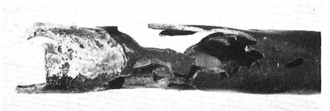
FIG. 7—POLYTHENE-SHEATHED CARRIER-FREQUENCY CABLE ATTACKED BY TERMITES ( MACROTERMES BELlicosus )
