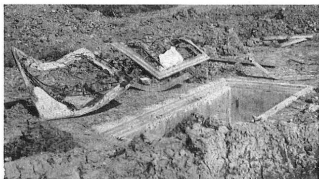
SURFACE JOINT-BOX DAMAGED BY LEVELLING MACHINE
