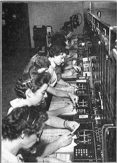
OVERSEA SWITCHBOARD IN WHITE PLAINS, NEW YORK, WHERE UNITED KINGDOM-UNITED STATES CIRCUITS TERMINATE.
