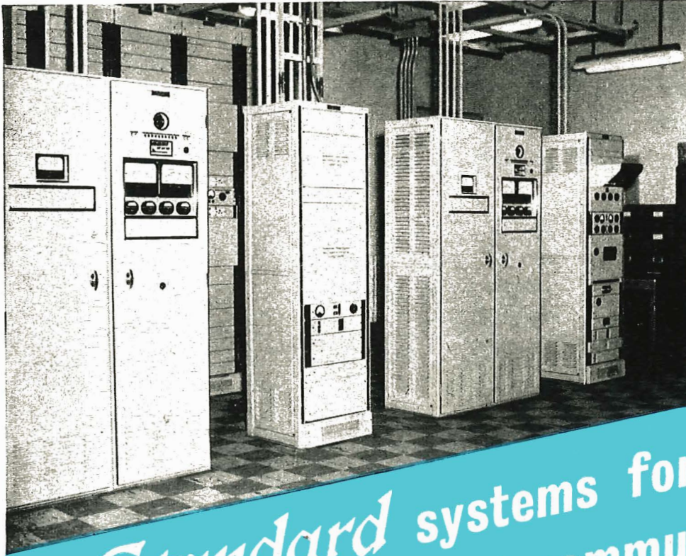
Submerged repeater power supply cubicles at Sydney Mines. Cable terminal cubicle is shown at centre.
