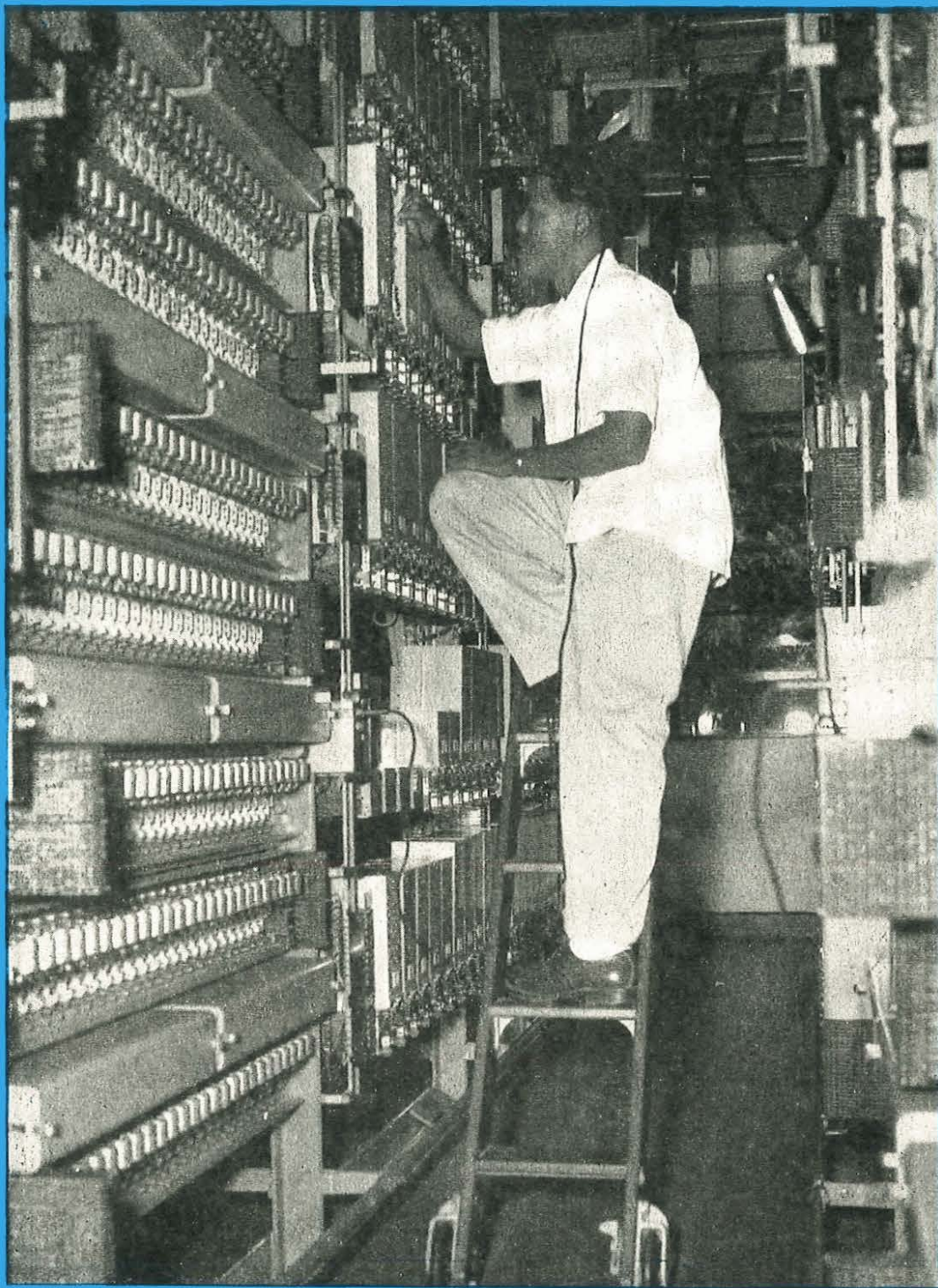
Local technician at work on the new exchange at Kuching — the first exchange to use SE50 Selectors in S.E. Asia.
