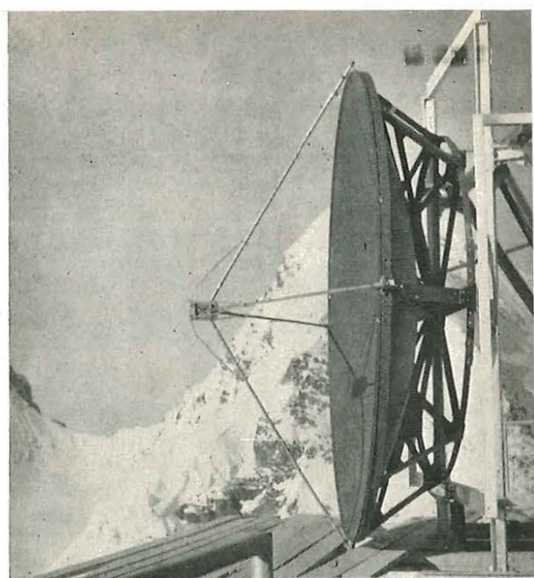
Snow and ice failed to delay the rapid installation of the G.E.C. aerial which faces Chasseral at the Jungfrauoch.
