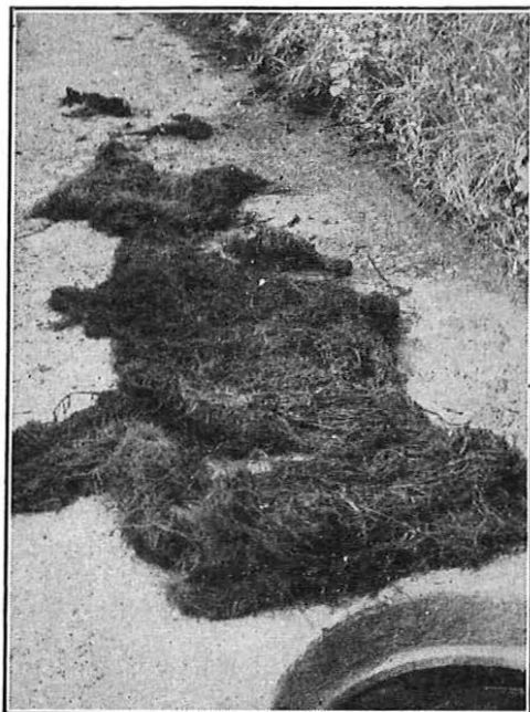
ROOTS REMOVED FROM MANHOLE.
