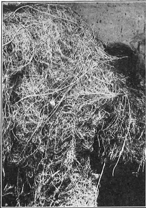
ROOTS GROWING IN MANHOLE.
