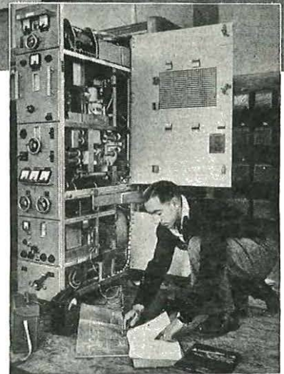
A member of the New Zealand P. T. & T. staff making adjustments during installation.
