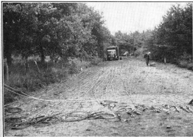
FIG. 5.—P.O. CABLES AND WIRES PREPARED FOR RAPID CHANGING BETWEEN TESTS.
