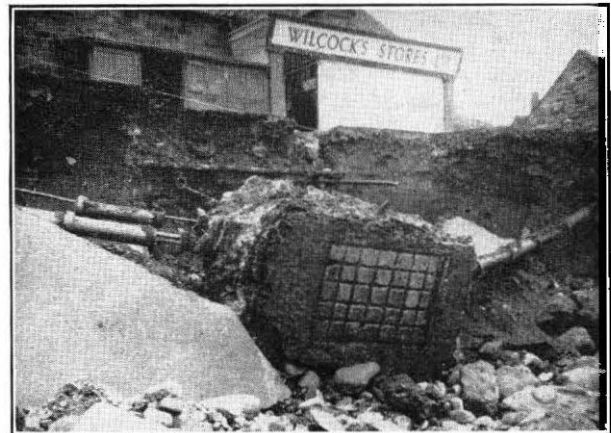
THE JOINT BOX SUSPENDED ON CABLES.
