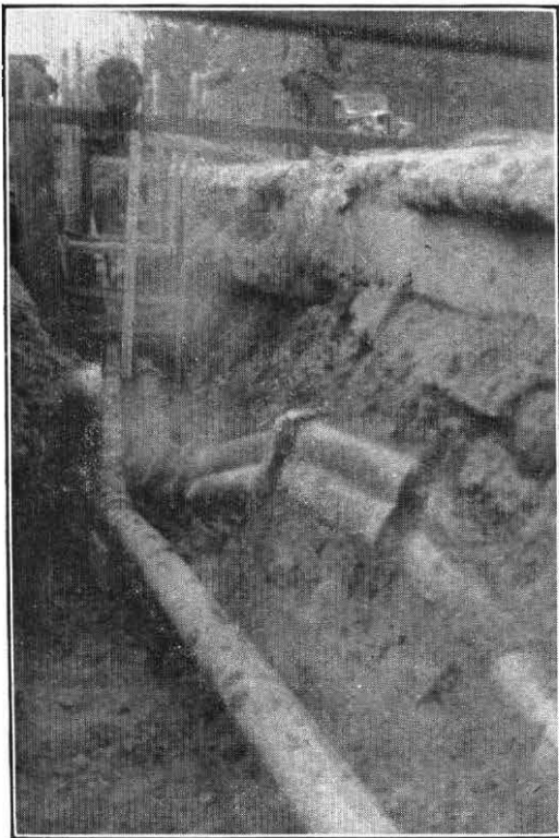
U.G. CONDUIT DISPLACED BY LANDSLIP.
