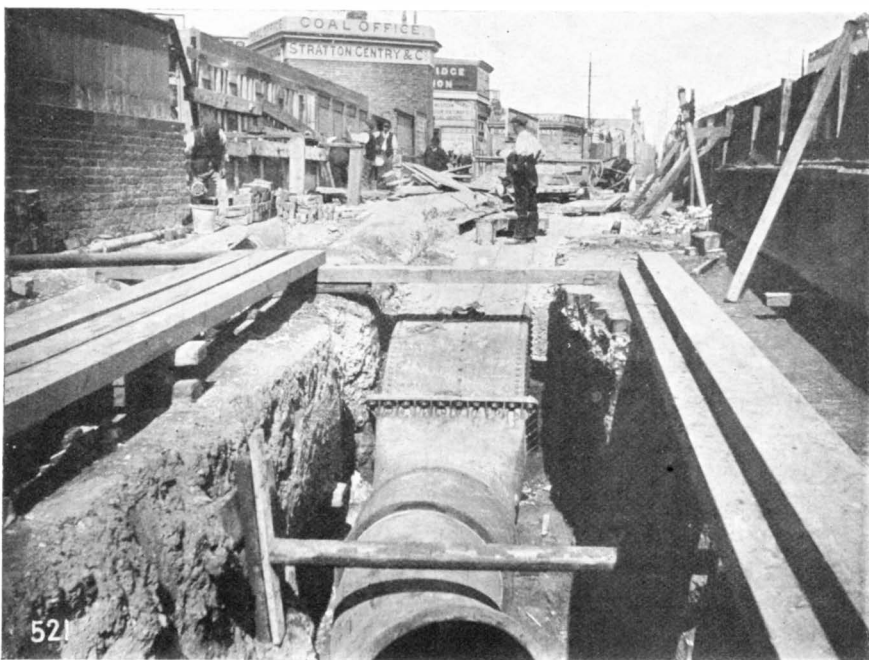
I.—NORTH SIDE. NEW PIPE MAY BE DISCERNED AT THE FOOT OF THE WALL IN LEFT FOREGROUND. THE SECOND IS UNDERNEATH IT. REMAINDER MAY BE SEEN IN DISTANCE.
