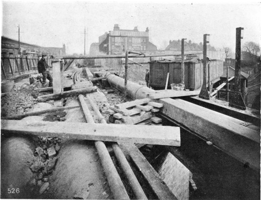
6.—SOUTH SIDE. SHOWS PIPES BEFORE REMOVAL. INTERMEDIATE BOX NEAR VERTICAL WATER PIPE.
