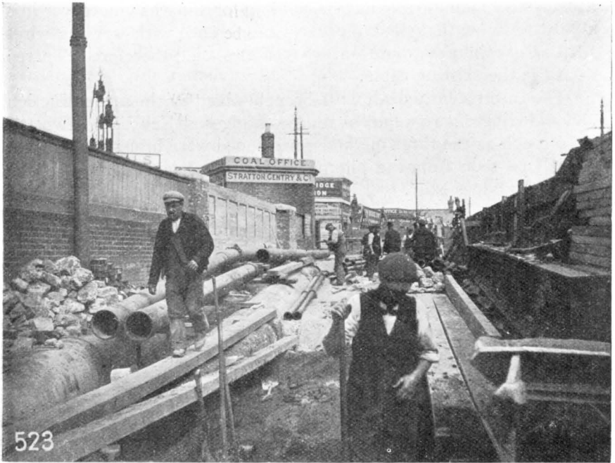
3.—NORTH SIDE. INTERRUPTION CABLE WAS SUSPENDED FROM TOP OF COAL OFFICE TO FARTHER TRAMWAY STANDARD.
