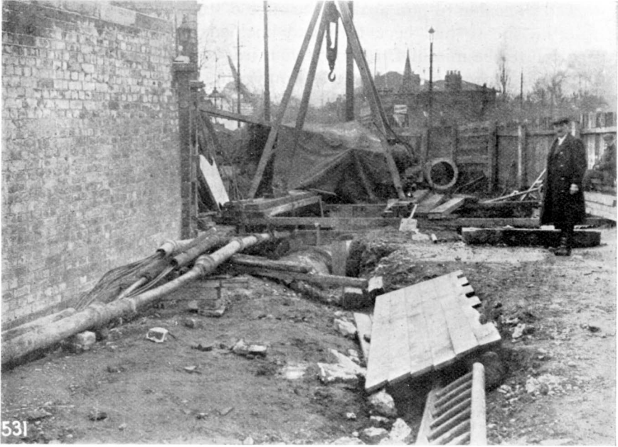
10.—SOUTH SIDE. SHOWS PIPES AFTER REMOVAL WITH BENDS CUT OUT. THE MIXING BOARD COVERS APPROXIMATELY THE ORIGINAL SITE.
