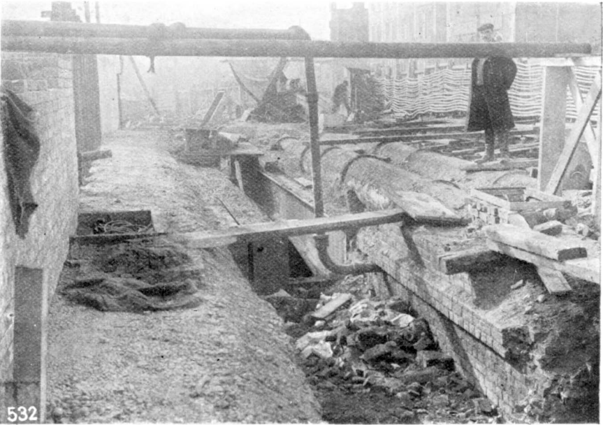
11.—SOUTH SIDE. SHOWS NEW INTERMEDIATE BOX. FRAME OF OLD BOX CAN BE SEEN ON OLD SITE. TRAMWAY INTERRUPTION CABLES IN BACKGROUND.
