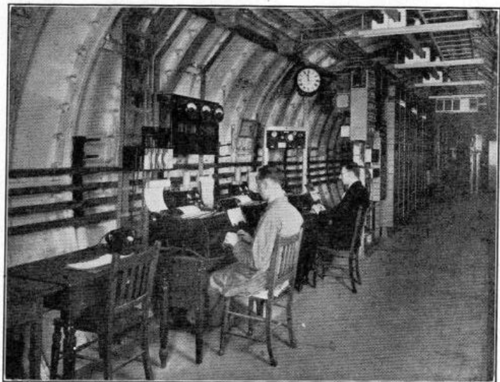
FIG. 6.—V.F. TELEGRAPH EQUIPMENT IN DEEP-LEVEL PROTECTION.
