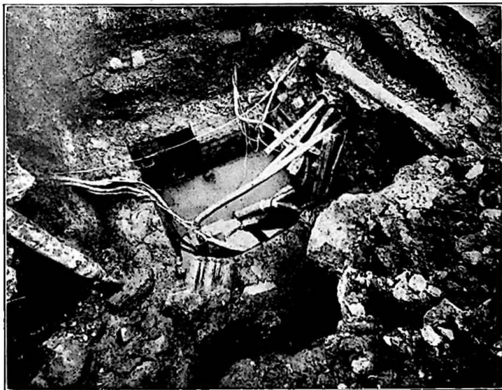
FIG. 4.—DAMAGE TO UNDERGROUND PLANT (BRIXTON, LONDON)
