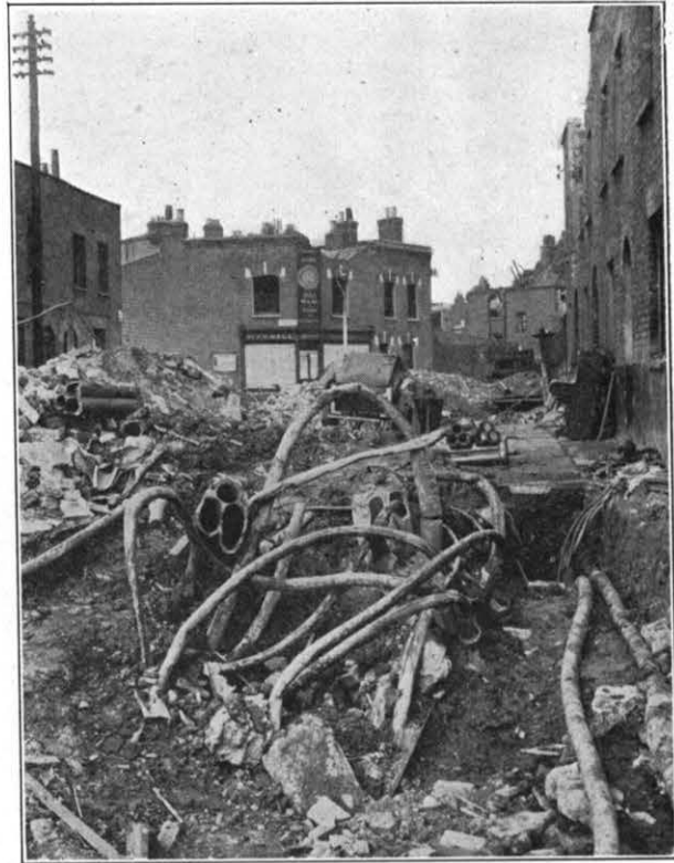
FIG. 2. DAMAGED UNDERGROUND CABLES.
