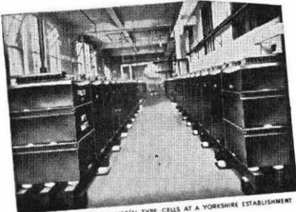
TWO ALTON BATTERIES OF JUV27/41 TYPE CELLS AT A YORKSHIRE ESTABLISHMENT
