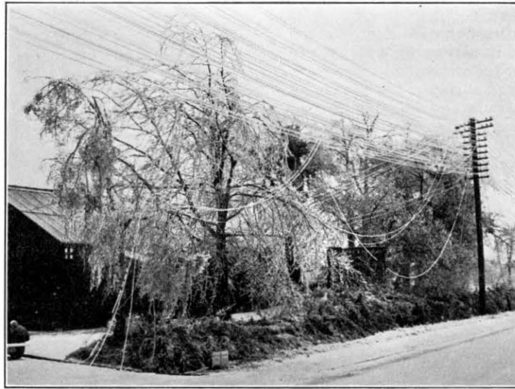
FIG. 11.—FALLEN WIRES ON THE SOUTHAMPTON-WINCHESTER ROUTE.
