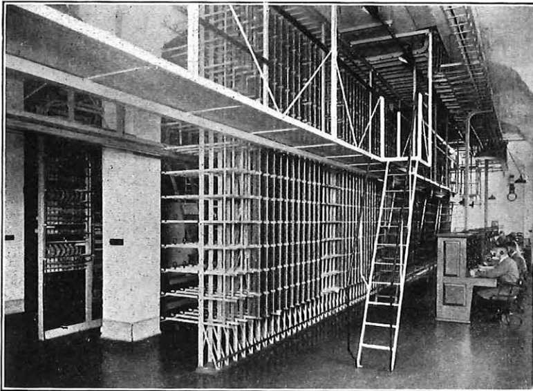
FIG. 3.—THE MAIN DISTRIBUTION FRAME.
