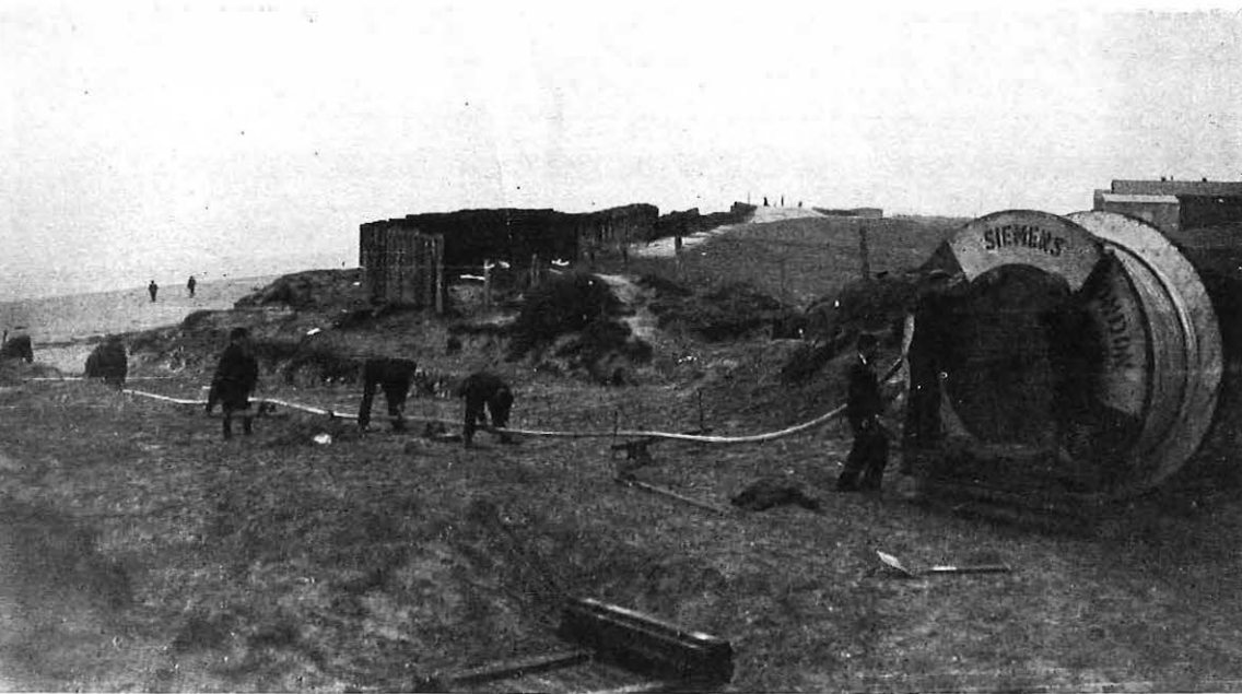
CABLE ACROSS AN ESTUARY
