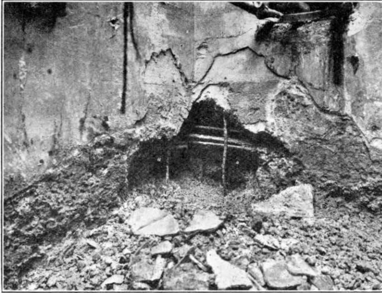
FIG. 3.—FURTHER EFFECTS OF SULPHATE CORROSION.
