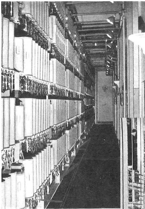
Final Selector Racks, Norte.
