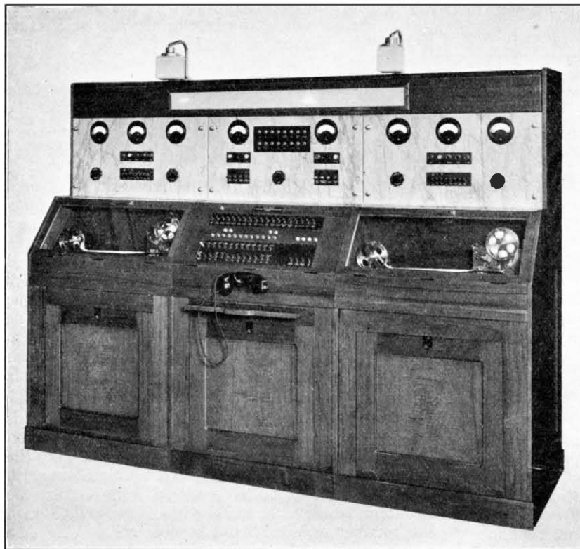
FIG. 6.—STATION EQUIPMENT AT HEADQUARTERS, LAMBETH.
