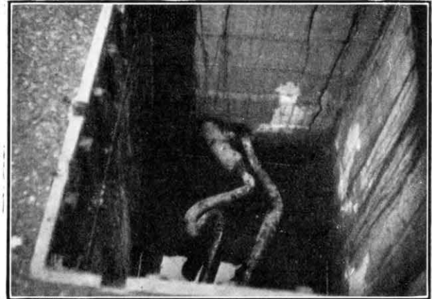
FIG. 2.—VIEW OF MANHOLE WHERE CREEPAGE HAS OCCURRED.
