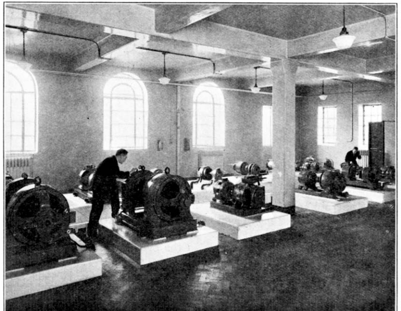
FIG. 3.—GENERATOR ROOM—CENTRAL BUILDING.
