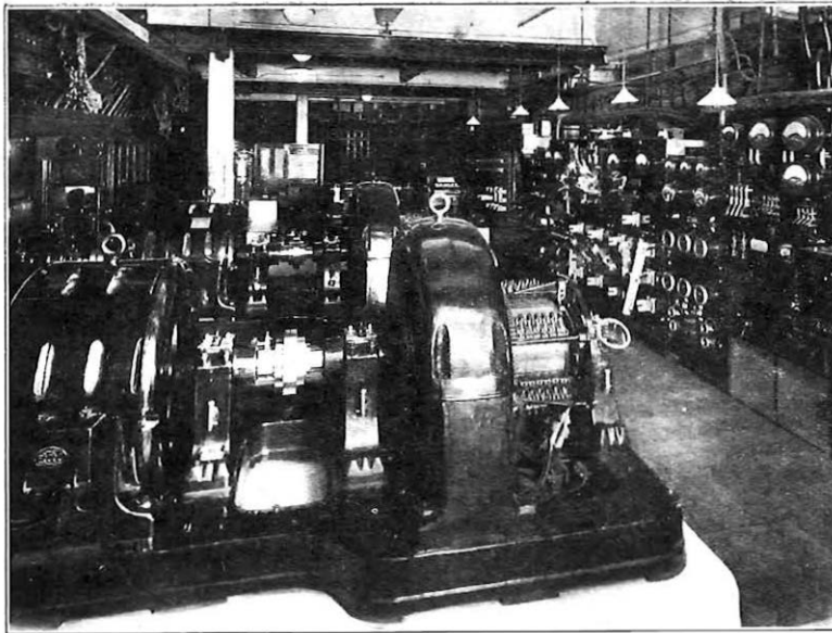
FIG. 3.—GENERAL VIEW OF POWER PLANT.
