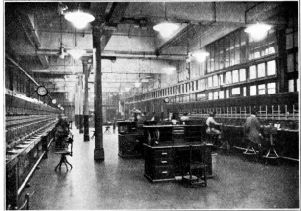
FIG. 4.—TELEPHONE TRUNK SWITCHROOM.
