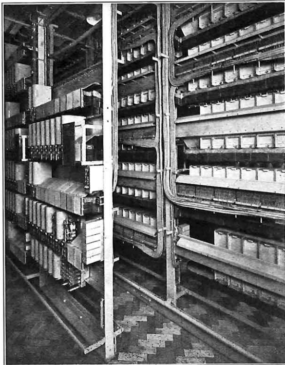
FIG. 3.—SECOND SELECTOR RACK, SHOWING CONTROL RELAY-SETS.
