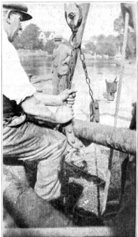
FIG. 5.—PIPE IN STIRRUP SUPPORT.
